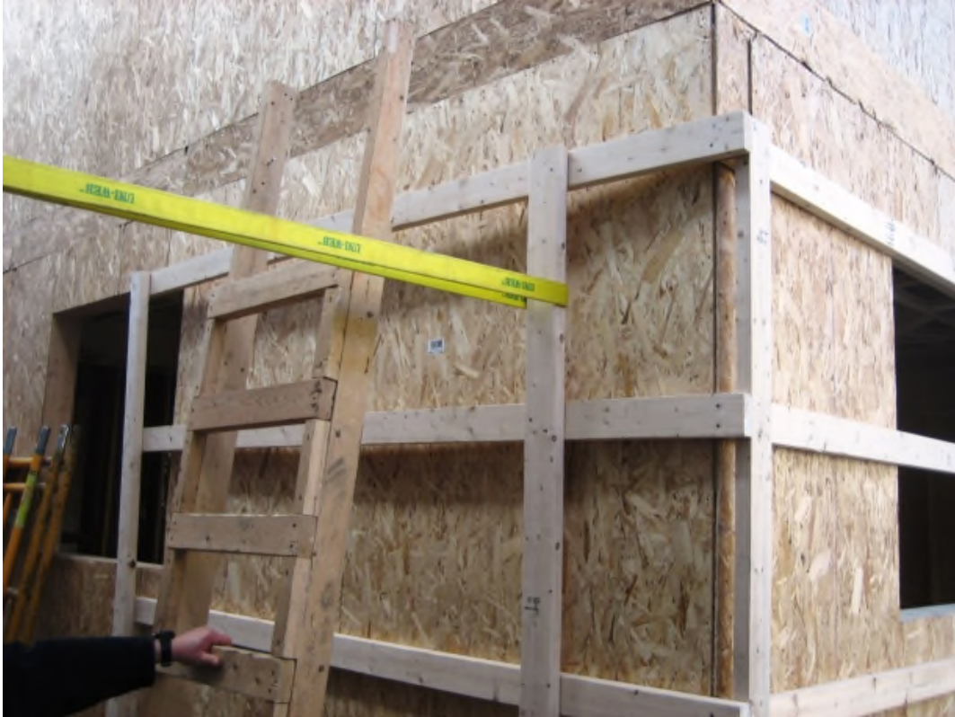
Figure 3: A line was attached to the mid-point of the top- and mid-rail to generate pulling forces on the guardrail.
