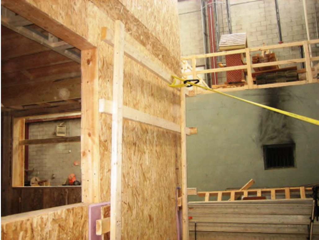
Figure 3: A line was attached to the mid-point of the top rail to generate pulling forces on the guardrail.
