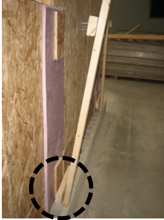
Figure 5: First trial - the post pulled out of the attachment point. Note the wrong installation of a 2x4 block at the bottom of the post. The maximum force was 306 lb.
