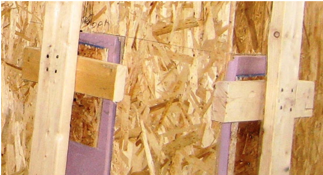
Figure 2: Four (4) 3/4 inches spiral nails were used to attach the guardrail post to the frame of the house with foam insulation.
