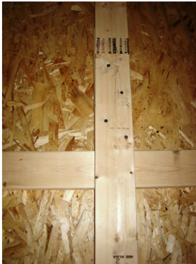
Figure 2: Four (4) spiral nails were used to attach the guardrail post to the frame of the house.
