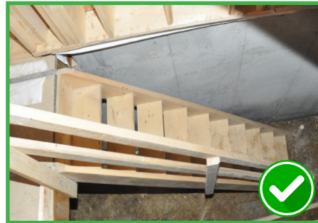
Properly sized and supported stairs
