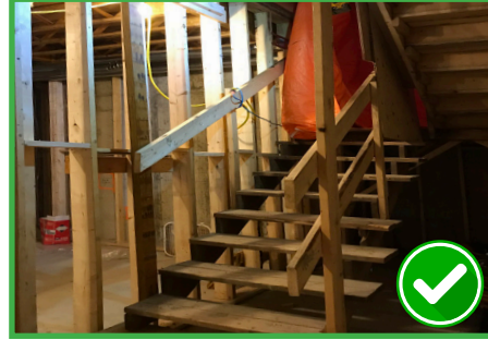
Bottom of stairway secured with uprights attached to stringers (at bottom) and floor joists (at top)
