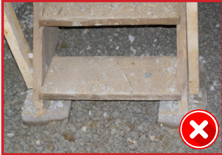
Bottom of stairway is not properly secured to floor
