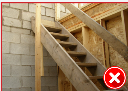
Stairway is poorly located (cannot end at a wall)
