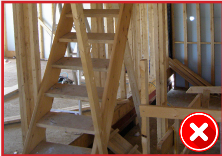
Stairway stringers are installed above maximum slope
