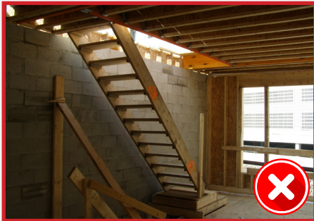
Stairway is too short and installed above a floor opening
